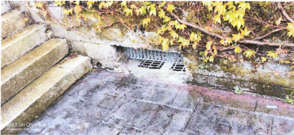
Drain at base of Granite Steps
