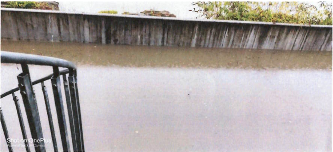
Proposed Walkway - Flooding
